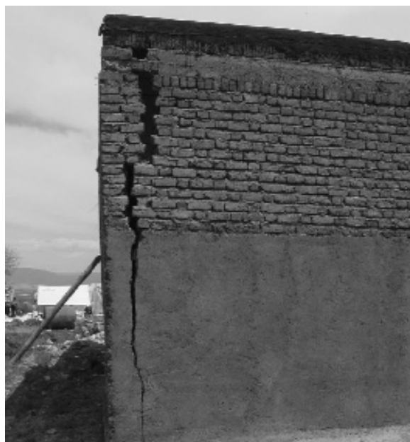
Fig. 1 Vertical crack in confined masonry wall due to out-of-plane action of other wall during Silakhor earthquake
