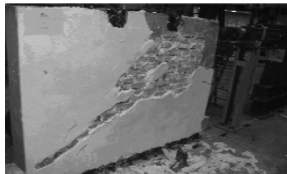
Fig 13 Separation of plaster due to crack formation in specimen B at last loading step
