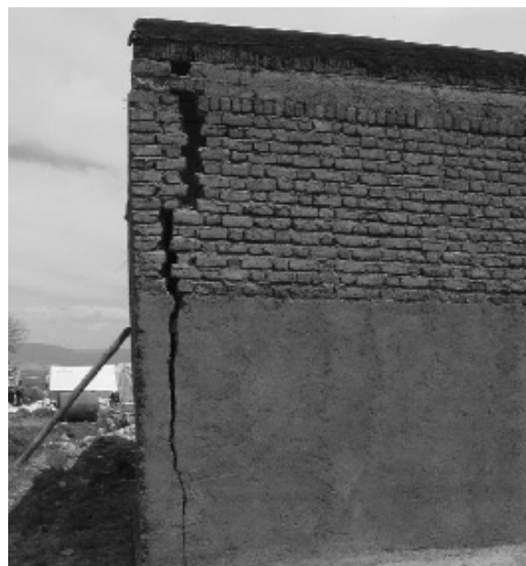
Fig. 1 Vertical crack in confined masonry wall due to out-of-plane action of other wall during Silakhor earthquake
