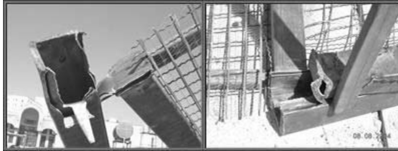
Fig.7 Destruction of beam to column moment connection
