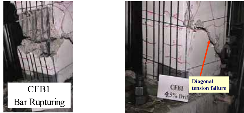
Fig.4 Observed Damages in Beam CFB1
