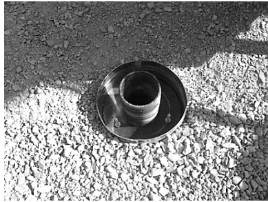
b. backfilling the sleeve with the excavated soil at the considered density
