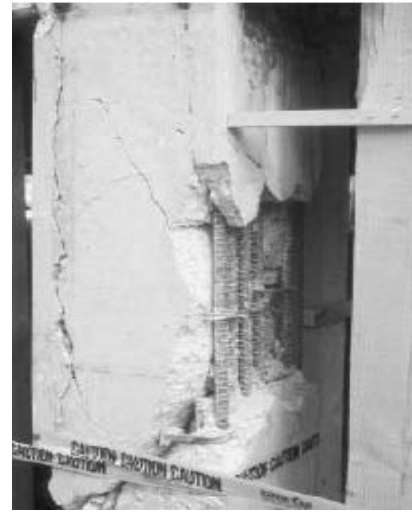
Fig.2 Failure of lap splice due to insufficient splice length and widely spaced ties with 90° hooks (Northridge-1994)
