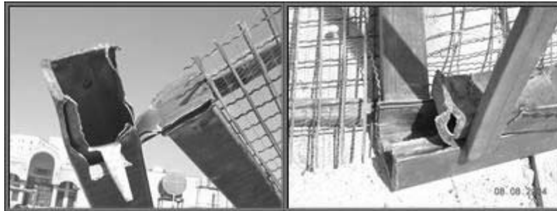
Fig.7 Destruction of beam to column moment connection
