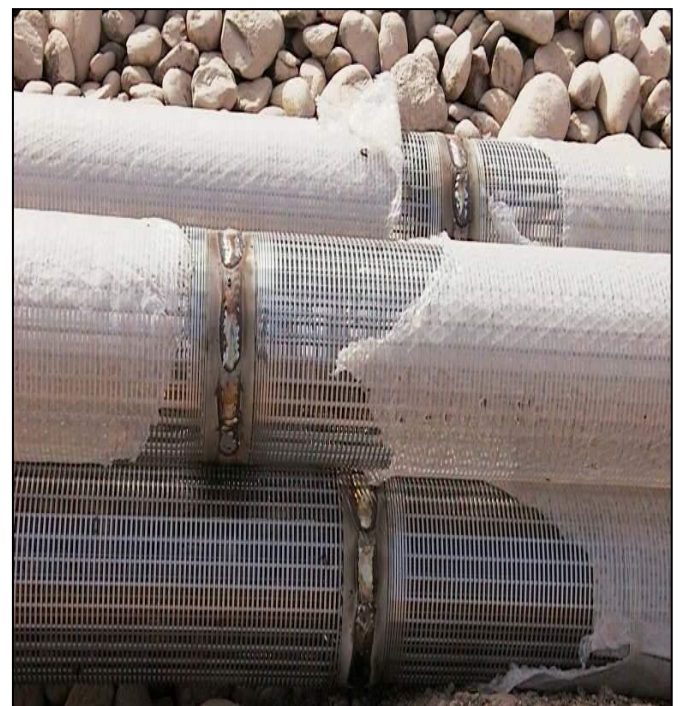
Fig. 9 Picture showing the arrangement and size of the well screens used for the new relief wells at the Karkheh dam
