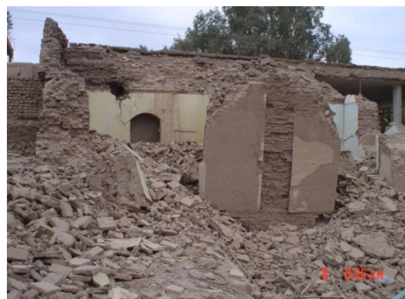
Fig. 1 A view of one sample destroyed adobe house after Bam earthquake
