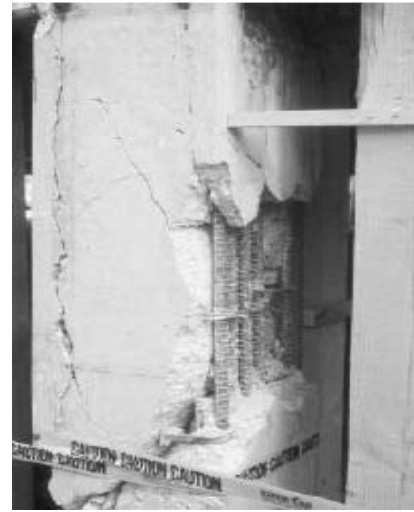
Fig.2 Failure of lap splice due to insufficient splice length and widely spaced ties with 90° hooks (Northridge-1994)
