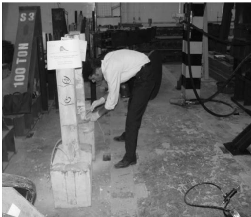
Fig.8 Cleanig surface of the damaged columns
