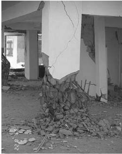
Fig.1 Failure of lap splice due to widely spaced ties with 90° hooks (Izmit-1999)
