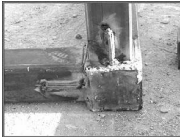
Fig.8 Using end plates and dowel plates in beam to column moment connections
