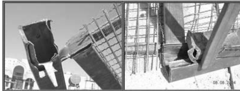
Fig.7 Destruction of beam to column moment connection
