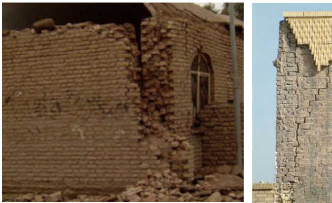
Fig. 11. Vulnerable wall-to-wall connection failed in Bam earthquake, Iran 2000
