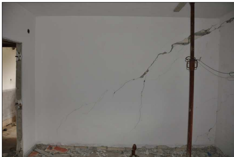
Fig. 37. Diagonal crack on a building in Bovino (Puglia, Italy)
