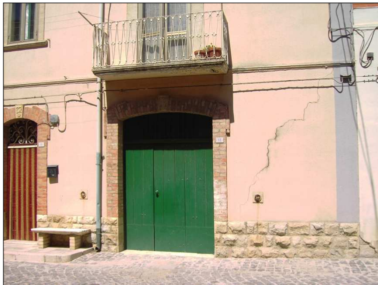
Fig. 36. Half arch-shaped crack on a building in Pietramontecorvino (Puglia, Italy)
